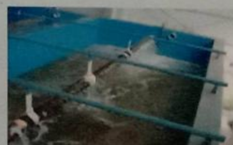
water collector tank
